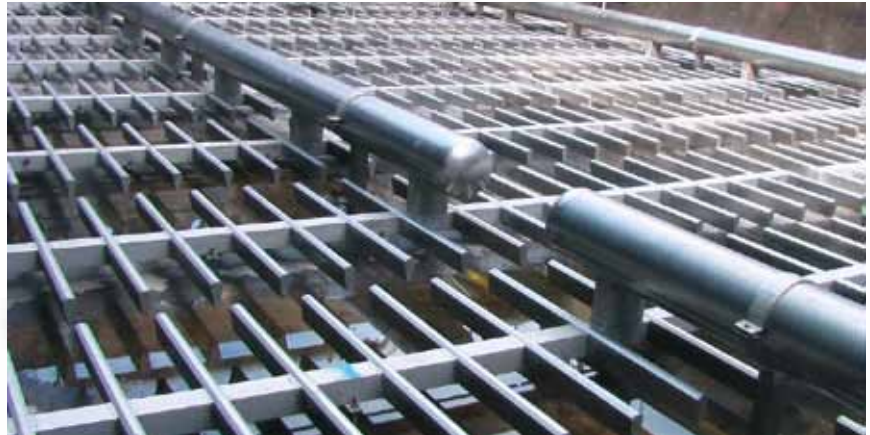
iCBA® aeration system in an industrial purification plant in Sweden (paper industry)
